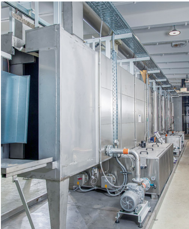
Inlet zone of the new pretreatment plant.
